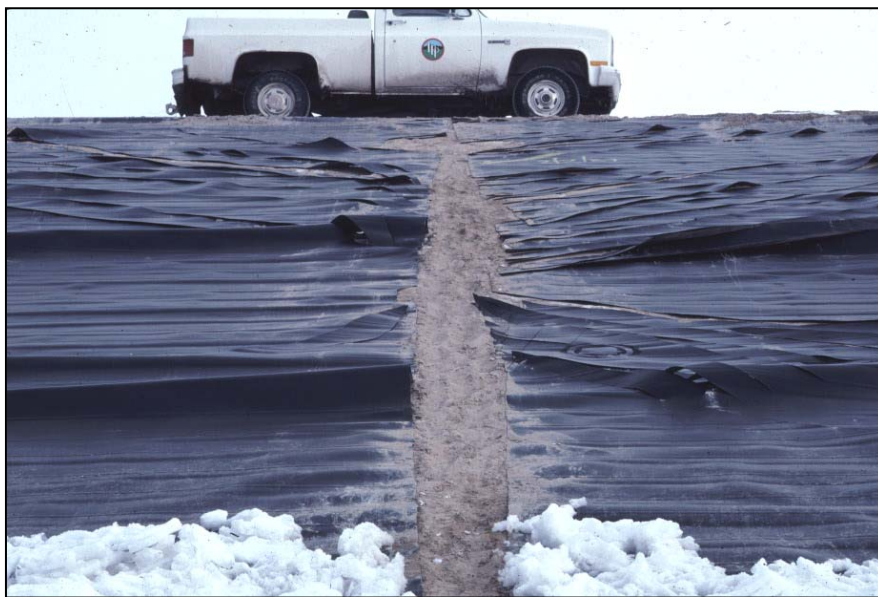
Fig. 1: Cracking of the geomembrane liner observed on the side slope of an empty geomembrane-lined reservoir after an extremely cold night. [Photo J.P. Giroud]
