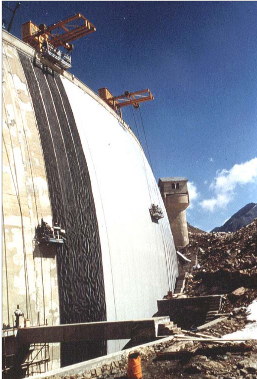
Fig. 13: Rehabilitation of a concrete dam, from left to right: concrete face repaired locally to smoothen surface irregularities, geonet drainage layer (black color), and geomembrane-geotextile composite with only the geomembrane component visible (light grey color). [Courtesy of D. Cazzuffi and A. Scuro]
