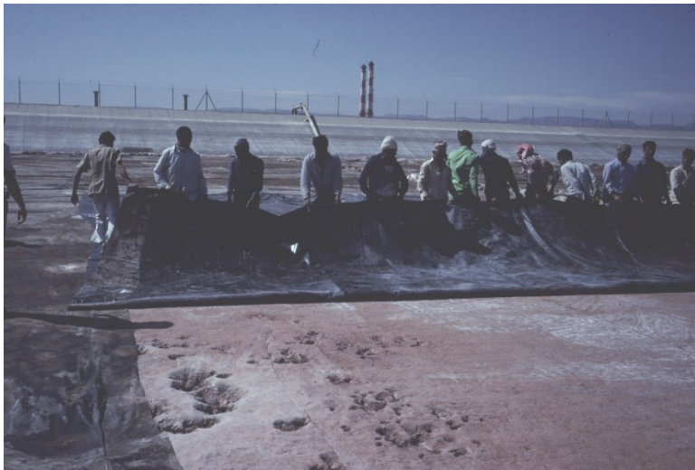
Figure 10. Cavities caused by several leaks of acid.
