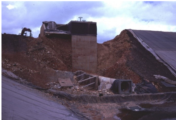
Figure 5. View of the failure area and the concrete structure.
