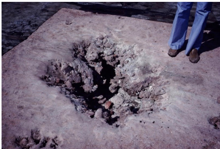
Figure 11. A large cavity over which the geomembrane burst.
